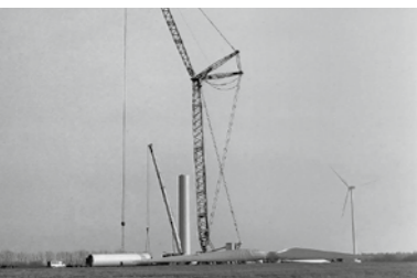
LARGE LATTICE MOBILE CRANE (Vestas V90 on 102 m tower)
